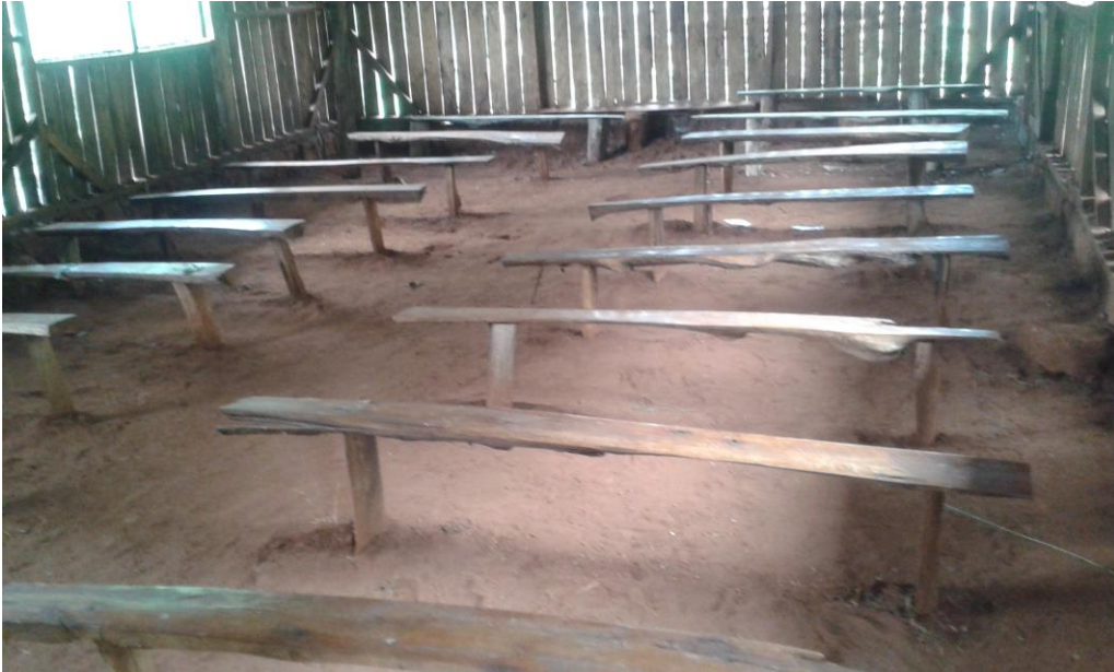
Dilapidated dining hall used for overflow classes
