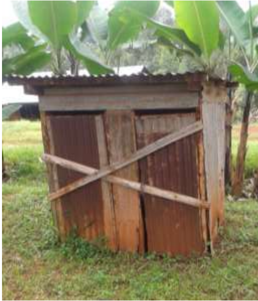
Latrines declared unhygienic by health department. Condemned as too risky for use
